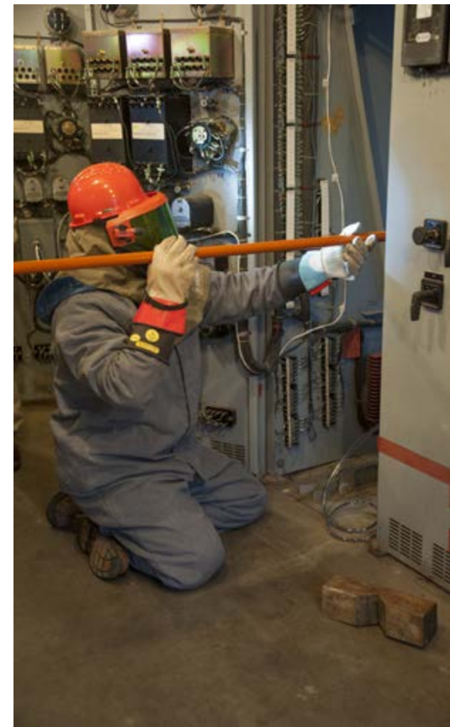
Y-12's Ed Crowder checks for absence of voltage in a 4,160-volt switchgear using the appropriate electrical personal protective equipment.
